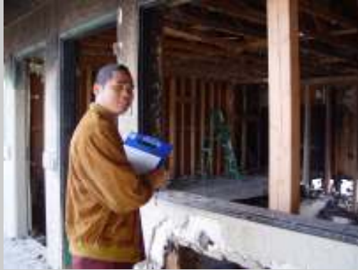
Ralph M., assisting during a "Fire Loss" investigation.
